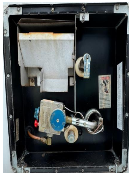
Hot Water Heater
